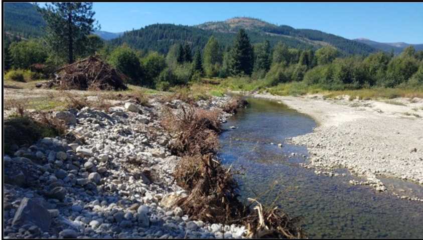
Streambank stabilization project on the Pack River incorporating large woody debris to enhance fish habitat.
